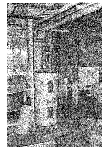
Figure 8: Electric Water Heater in Basement
